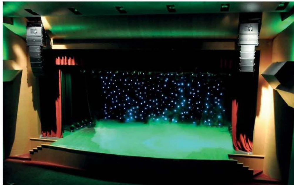
The system called for 12 DAS Audio Aero 12A line array cabinets flown in L-R hangs
