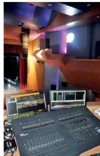
The lighting system is controlled by a Strand Lighting desk
