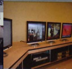
Control room at the Dead Sea Convention Center, Jordan, with MultiView full-matrix Cat5 switchers and local monitors, permitting full content-to-display flexibility. The system is tied into the CCTV security system. (Source: INTE)
