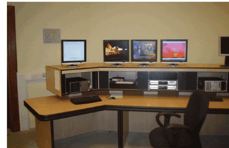
The control room monitors the content on all the displays throughout the site.
